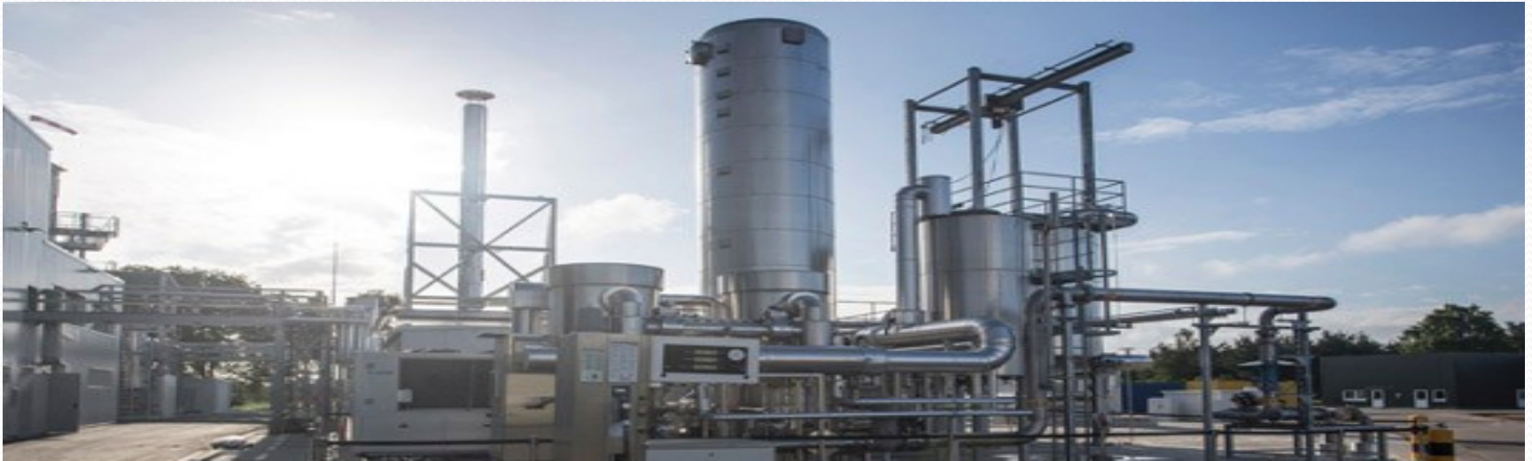
Audi Car Company 6 MW e-gas plant in Germany, begun in 2013.
